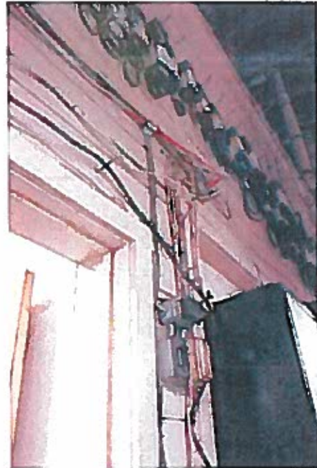
Wiring w/ Extension Cords
