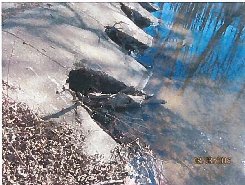
Debris at the inlet of Pipe 1.
