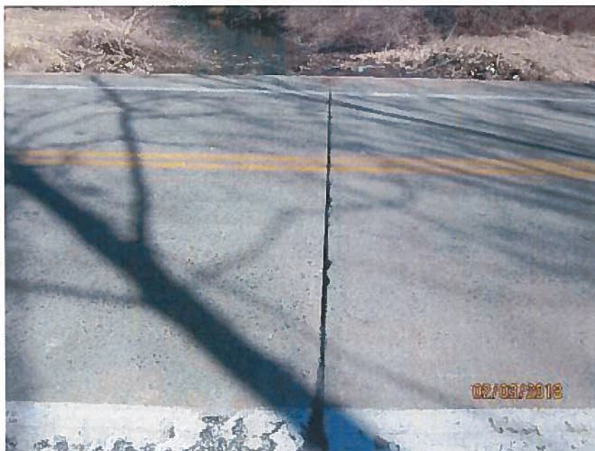
Joint between reinforced concrete slab over pipes and general condition of slab.
